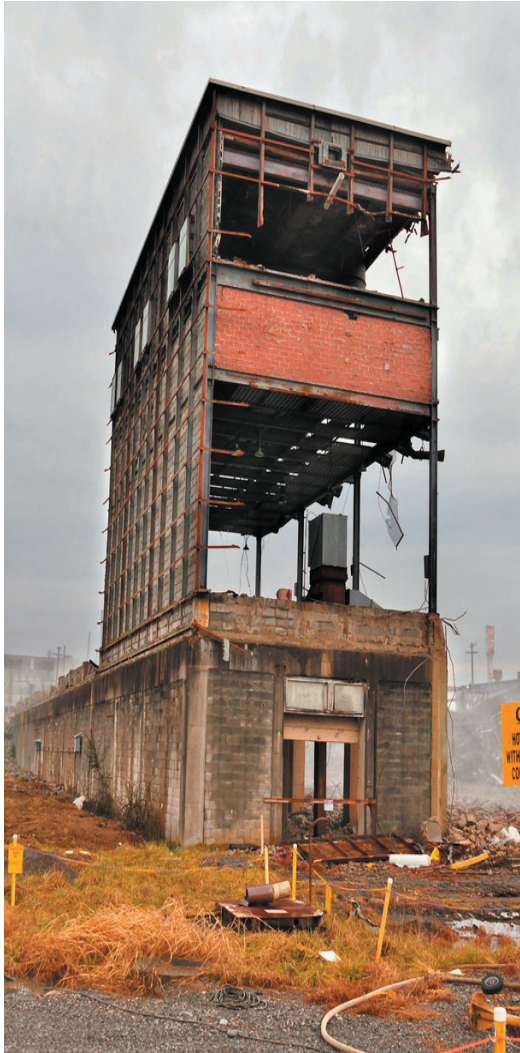
Remnant of the K-25 plant during the demolition of the east wing. See story on page 6.
