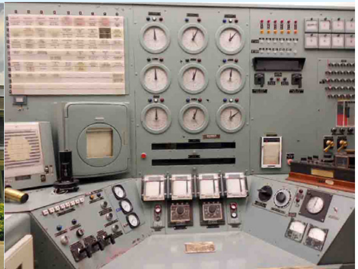
The control room of the B Reactor
